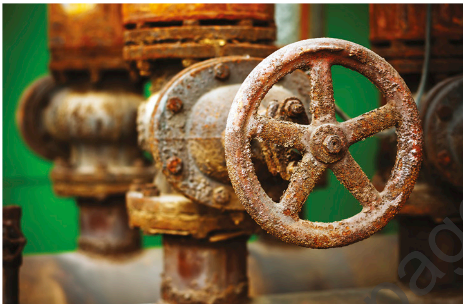
FIGURE 5.1.14 Corrosion is causing water to leak in these pipes in a pumping system.
